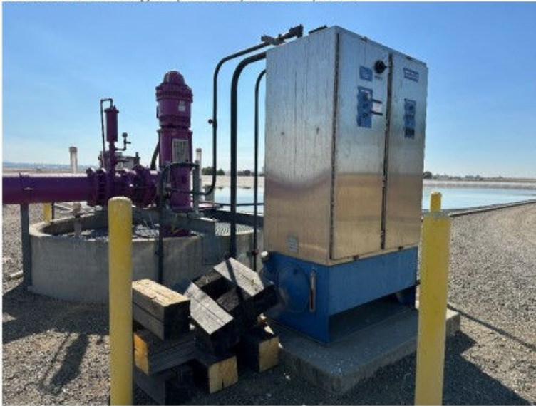
Photo 2. TSB Emergency Gate Hydraulic System
