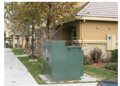
NOT PERMITTED: Transformers not screened from view and located adjacent to building entrances.
