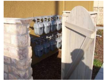
ENCOURAGED: Gas meters banked and located within an enclosure.
