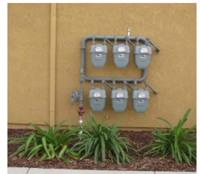
NOT PERMITTED: Gas meters not painted or appropriately screened.
